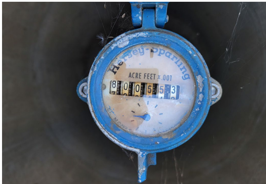
Figure 3-3. Corning Water District Meter
