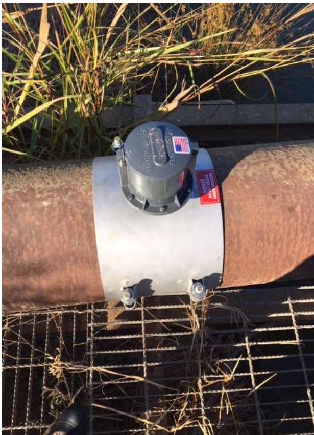
Figure 16. Flow meter installed in an in-flow pipe.
